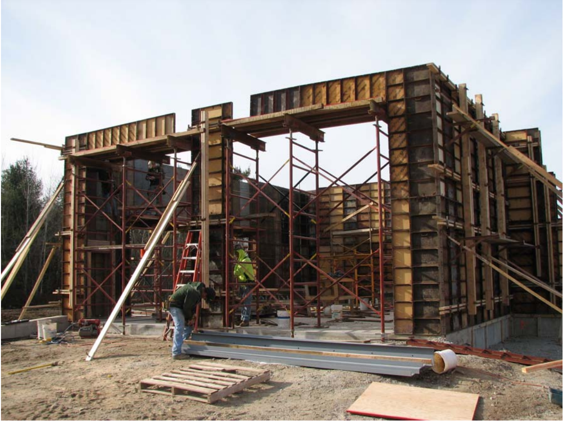
Fuel delivery area (walls not yet poured and no roof. Walking floor not installed.)
