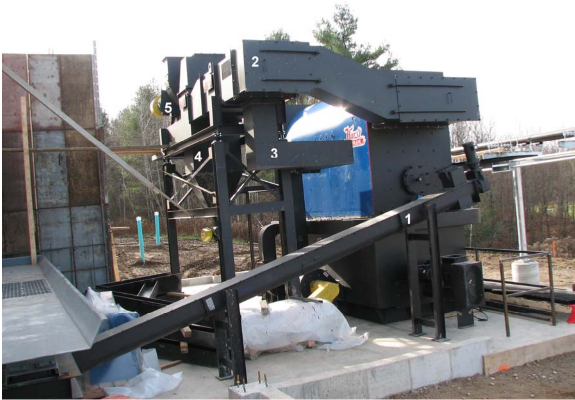
Hurst Boiler showing (1)fuel feed-in (not fully assembled), (2)exhaust gas heat exchanger for (3)pre-heated combustion air, (4)cyclone, (5) induced draft fan. No walls or roof yet.
